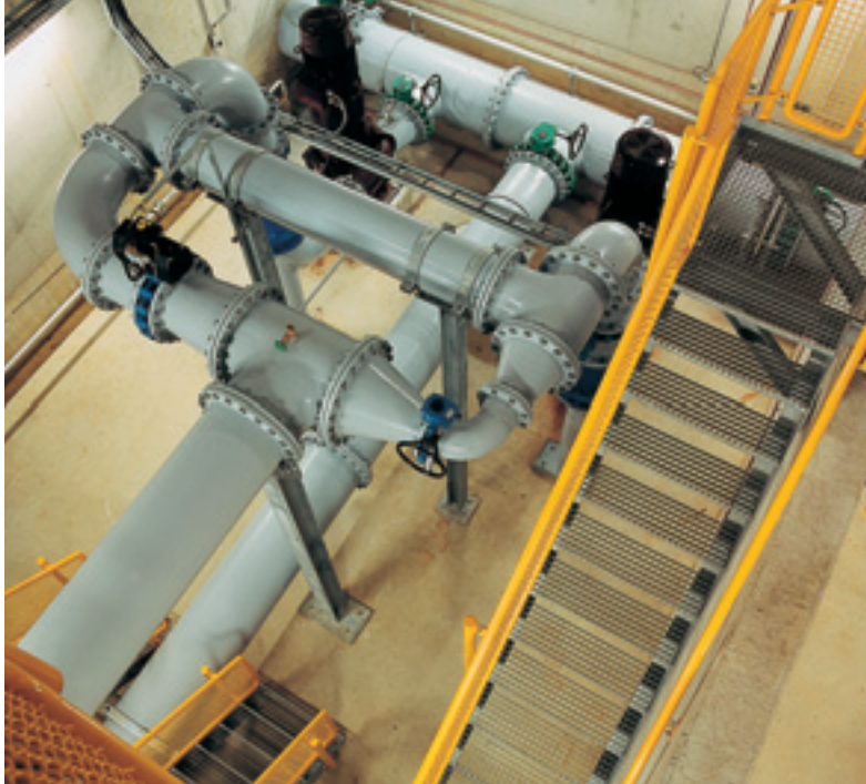
Potable water installation, Bergen op Zoom (NL)
