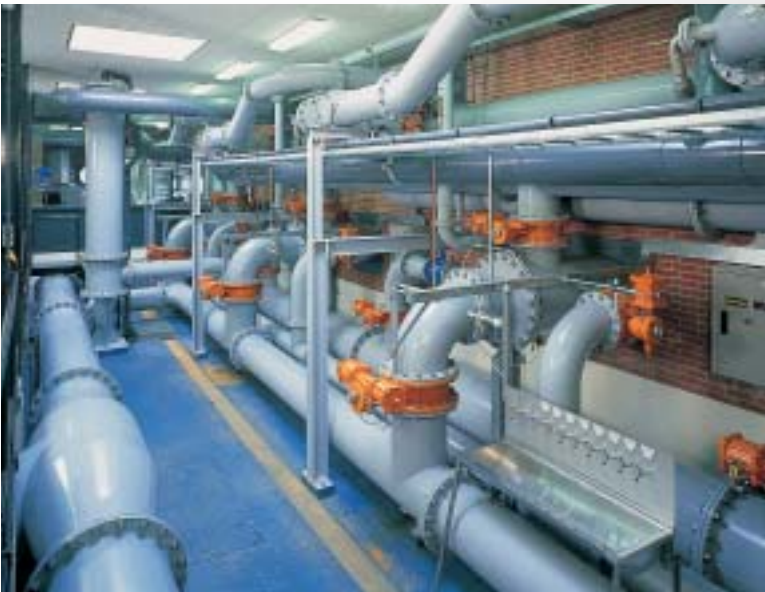
Potable water installation, Arnhem (NL)
