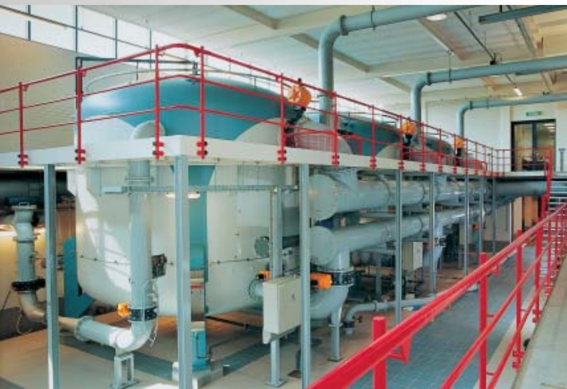
Potable water installation, Wierden (NL)
